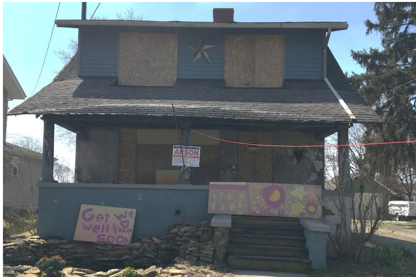
Fire damage to 203 Belle Avenue in Bellevue (Sandusky County).
