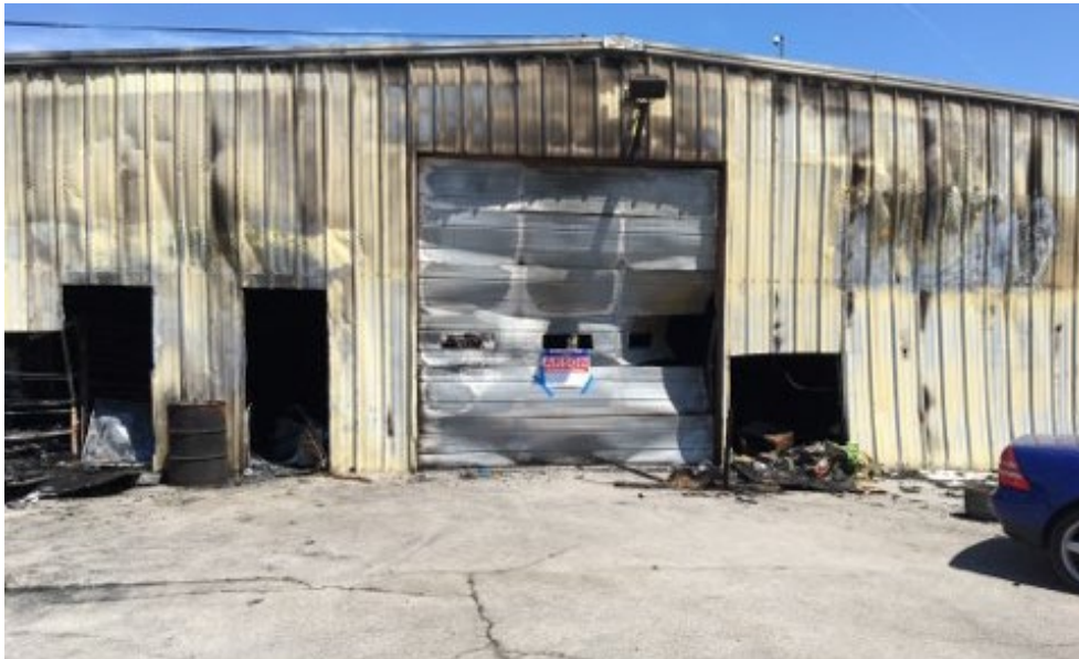
The scene of a fire at 8232 Fremont Pike in Perrysburg (Wood County).
