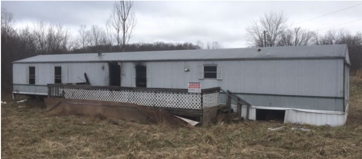
The scene of a fire at 16129 State Route 772 in Waverly (Pike County).
