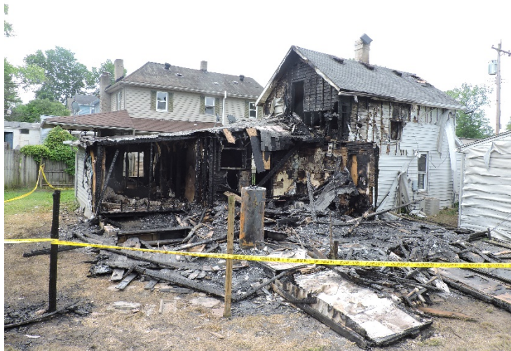
The scene of a fire at 127 W. 27 th Street in Franklin (Warren County).
