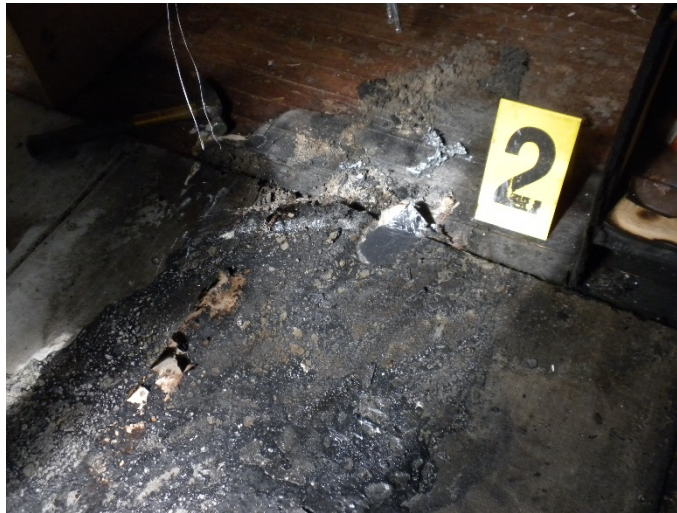
The scene of a fire at 4969 E. 84 th Street in Garfield Heights (Cuyahoga County).
