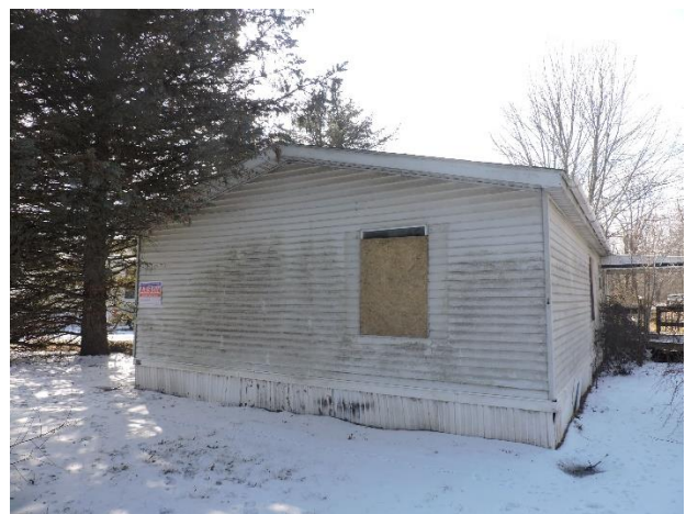
Fire damage to the home at 2170 S. Berkey Southern Rd., Lot 180.
