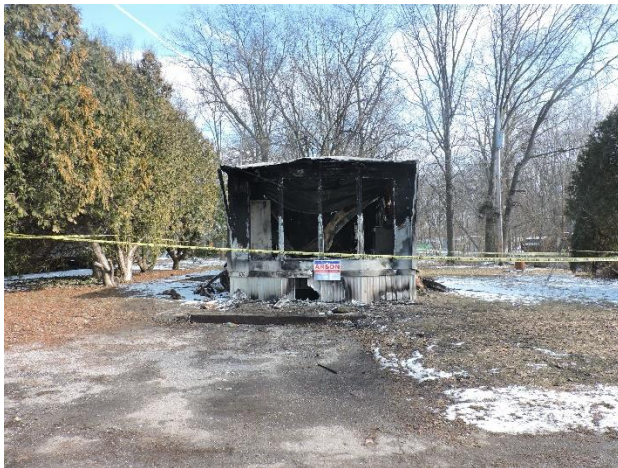
Fire damage to the home at 2170 S. Berkey Southern Rd., Lot 134.
