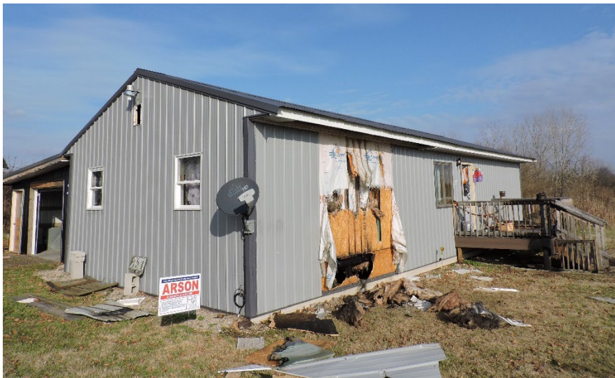
Fire damage to 26717 Old U.S. 35 in Chillicothe.
