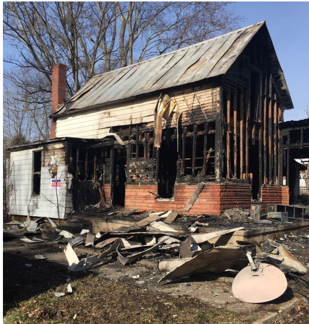
Fire damage to 92 Walnut Street in Peebles (Adams County).
